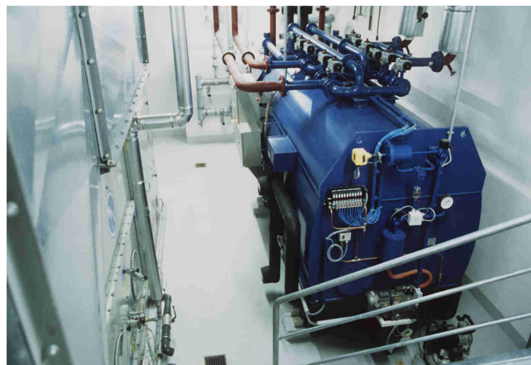
Figure 1: 70 kW Adsorption Chiller (GBU NAK 70), University Hospital Freiburg, Germany
